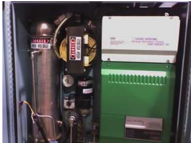
Figure 2: Ozone Generator Portion
