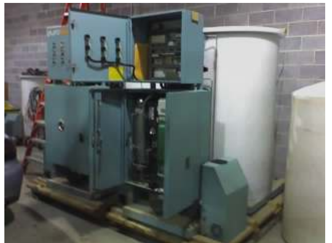
Figure 6: Systems and Controls on Skids
